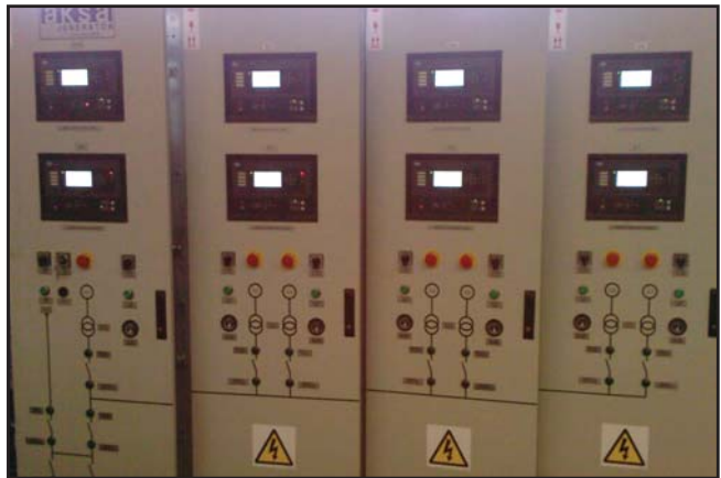
Multi Gen-Set & Multi Mains Paralleling System
