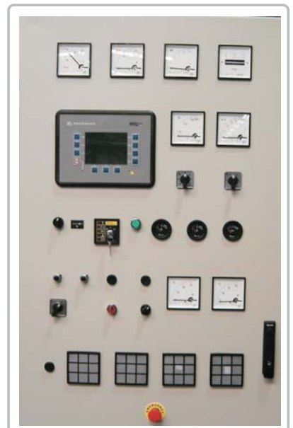
Control Panel with Woodward Easygen 3200
