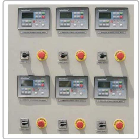
Multi Gen-Set & Multi Mains Paralleling System
